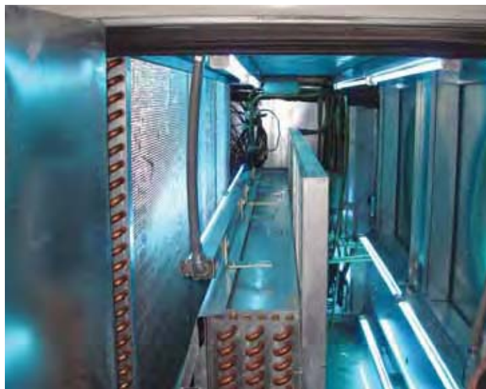
Eco-Care, a company specializing in pollution control and energy conservation, installed UVC lights, on a phased basis, in three air-handling units serving the ASPCA building in New York City.
