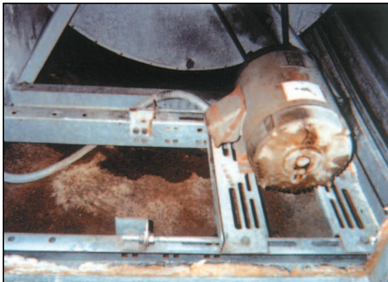
This air handler at Jennie Reid Elementary School shows a condition of mold and organic buildup similar to that at Rizzuto Elementary before UVC lights were installed.
