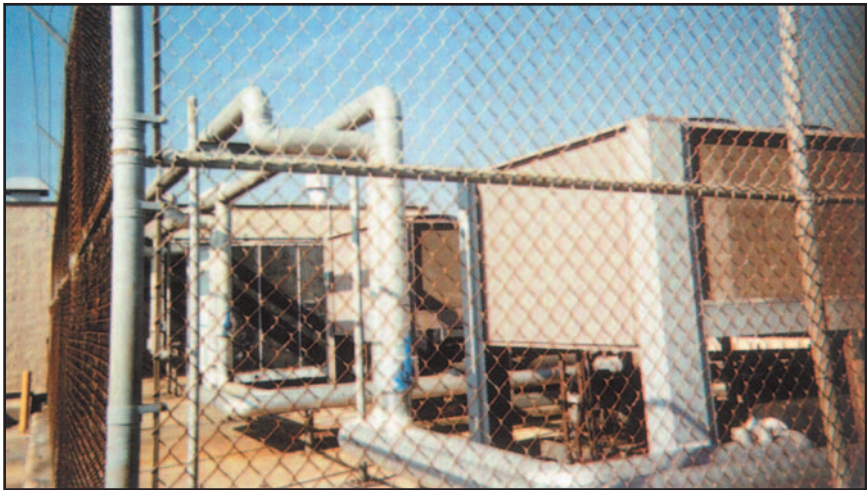
The chiller plant on the Jennie Reid Elementary school campus.
