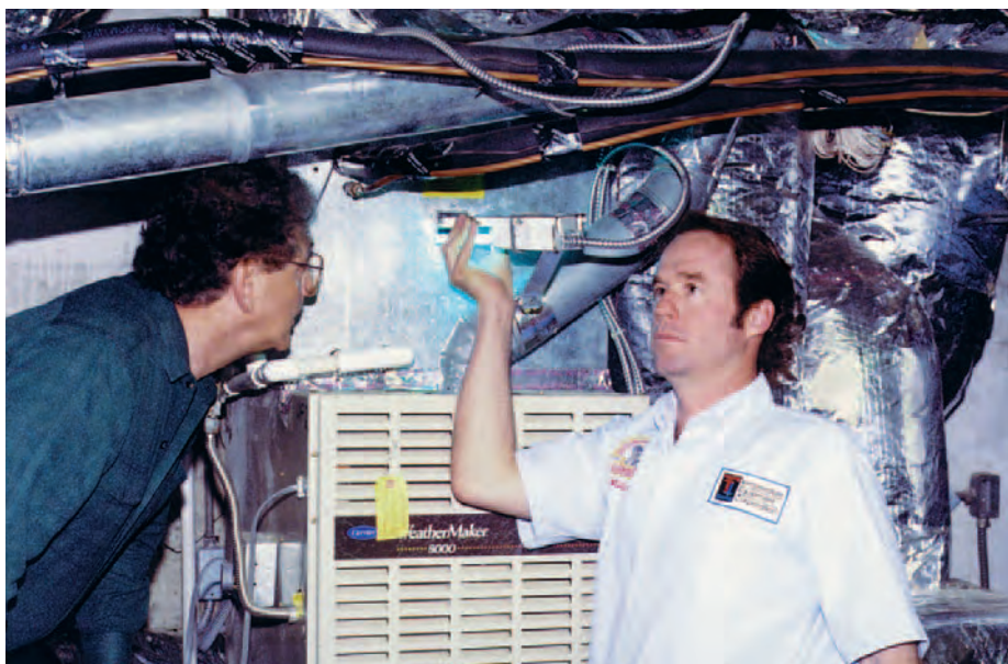
DR. ROBERT SCHEIR (left) looks on as Michael Holm installs a UVC Emitter in a residential a/c system.
