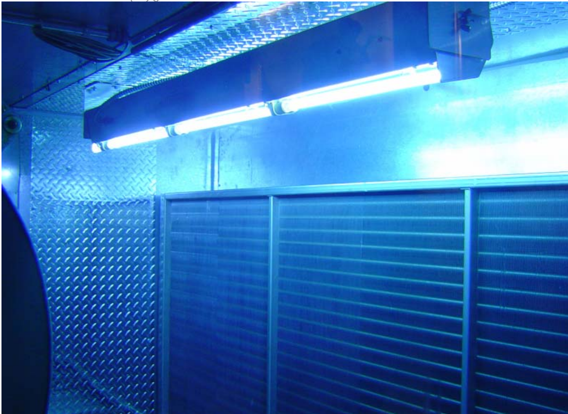
Figure 7: A UVGI system installed in front (upstream) of a cooling coil that sterilized the front face of the coil after two weeks of operation.
